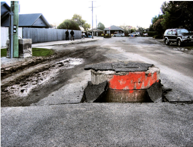
Photo Martin Luff BY-SA/2.0 The Darfield earthquake of September 2010 caused much damage in Christchurch, 40 km away. Vertical movement pushed this storm drain up through the road in Brooklands (northern Christchurch NZ).
