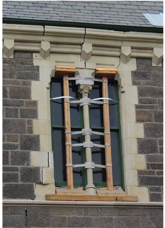
This 40 m long wall of the Christchurch museum “stretched” 100 mm as its foundations separated during the 2010 earthquake.
